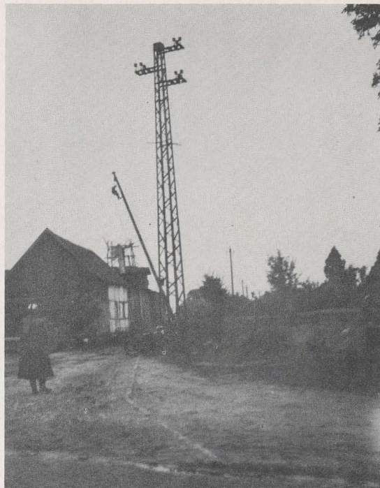
Most unusual picture of the trip was taken by Mrs. Miller in a small German village. The telephone pole has just broken away from the steel transmission tower, and the man strapped to it is apparently falling to his death. He broke the strap however, landed on the house, and escaped injury.
