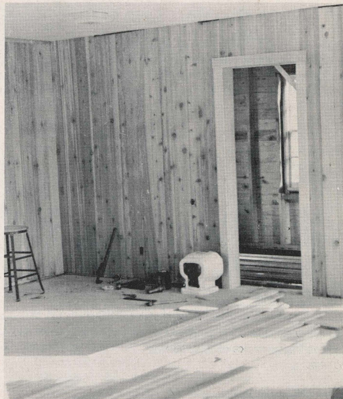
Interior of the building is not complete. It will contain a study room and library, a heating unit, and three engineering testing rooms.
